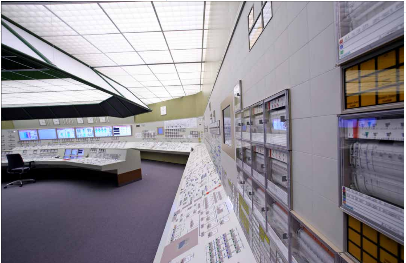
Kraftwerkswarte/Power Plant Control Room
